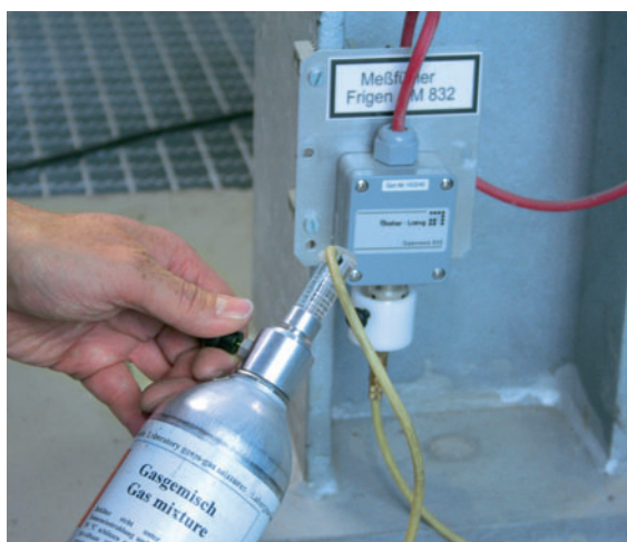
Figure 5: The function of a gas probe at ground level is checked by means of a test gas.
